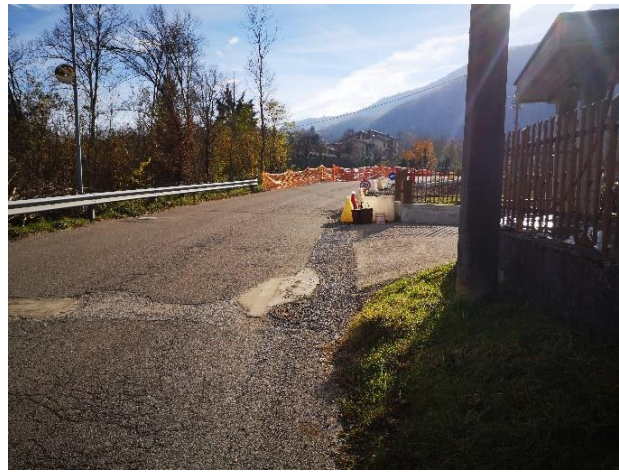
The road surface is asphalted, with some sections slightly damaged by roadworks.
